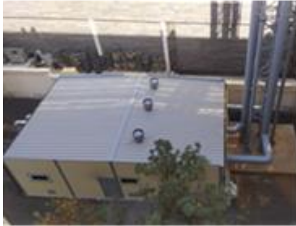
Individual campus heating system to reduce natural gas (Heating system based on electric heats and use solar energy )
