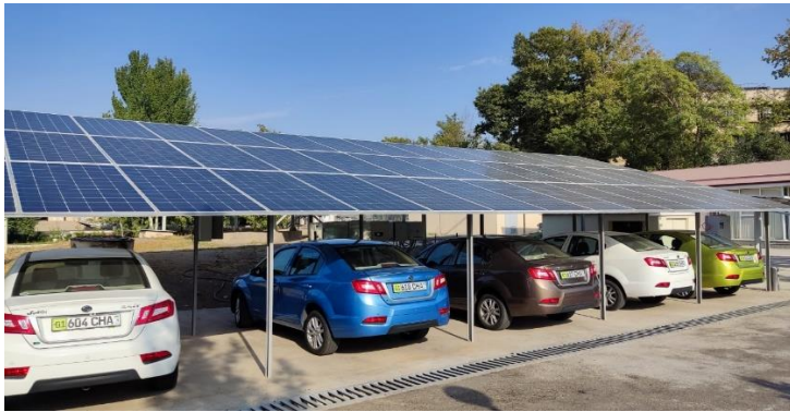
1. Charge parking (“TIIAME” NRU)
