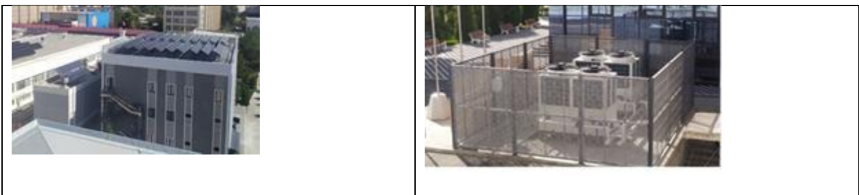
Solar absorption Air Conditioning system (“TIIAME” National Research Univeristy)
